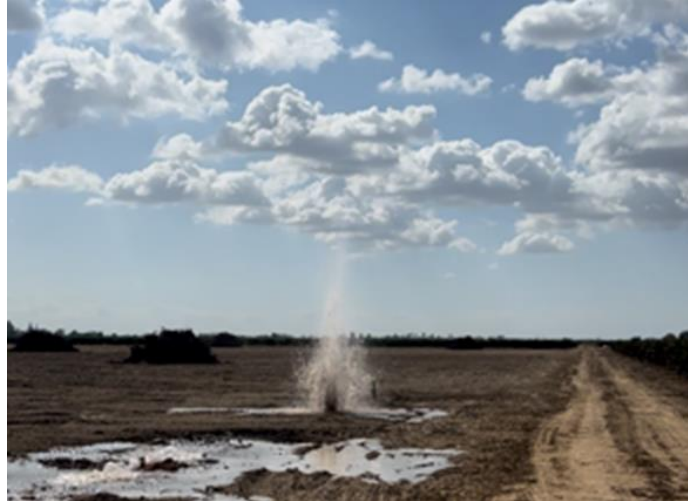
Air in the pipeline brings an Old Faithful Display to the Lakso Recharge Project
